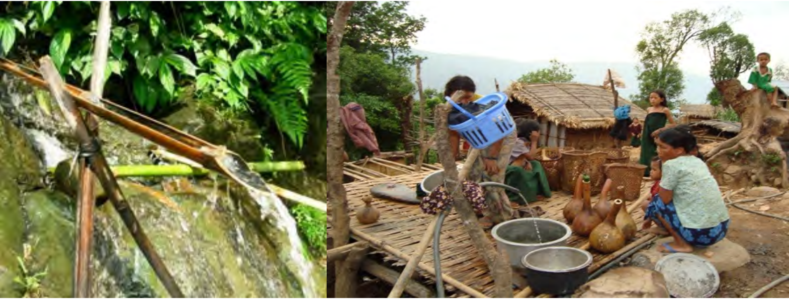
Bamboo-pipe (left) and plastic pipe used to bring water to community in Chin State (Photo: CHRO)
